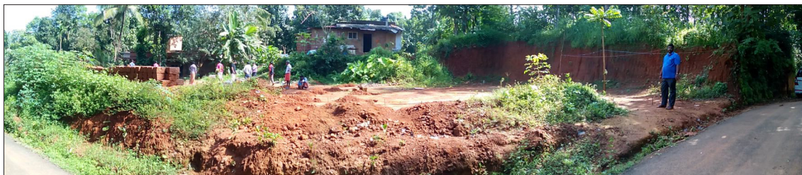
Fig. 2: Panoramic view of the soil pipe location at Mr. Sharif's land. Note the excavated loose laterite soil in the foreground.
