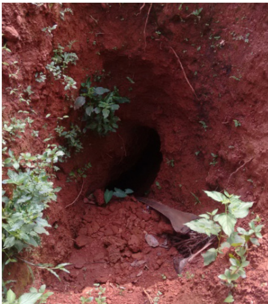
Fig. 3: Exposed view of the Soil pipe. Note the loose material at the mouth of the pipe.
