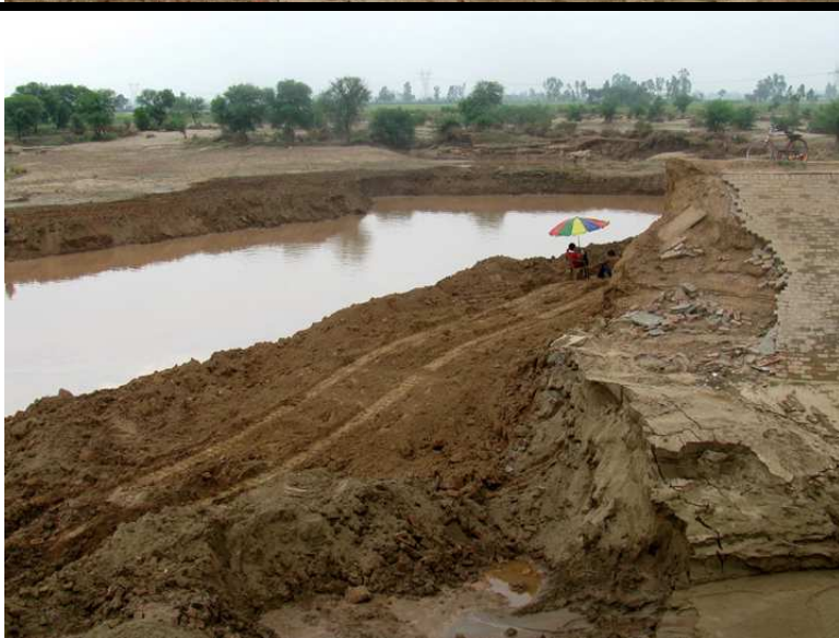
Supervision of repairing work near Tatiana village of Kaithal District in Haryana.
